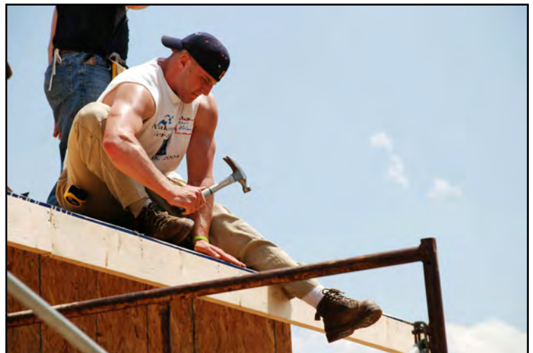
Senior health science/physical therapy major Kevin McCann works on the roof of the Habitat house on Foraker Avenue in Findlay.
