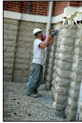
Far left, contractors lay sod in the residence halls courtyard. Left, the foundation of Old Main gets some tuckpoint work done. Photos by Anne Risser Lee.
