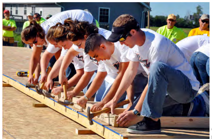
Student volunteers pound nails into the framework of a house to prepare for the wall raising.
