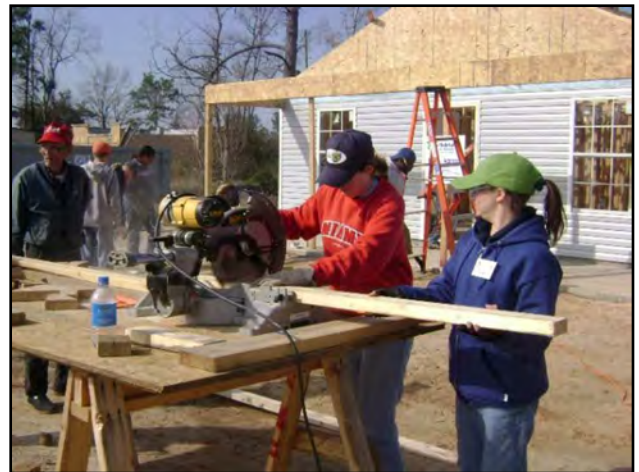
Chelsey Anglin (left) and Amy Lack (right) use a table saw to prepare a board for the house behind them. The students traveled to Biloxi, Miss., for a Habitat for Humanity Alternative Spring Break.
