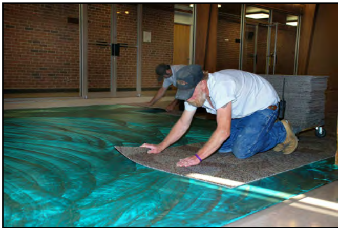
Randall Hertell, maintenance, helps lay new carpeting in the Alumni Memorial Union Multipurpose Room. The project is one of many to be completed by the Physical Plant this summer.
