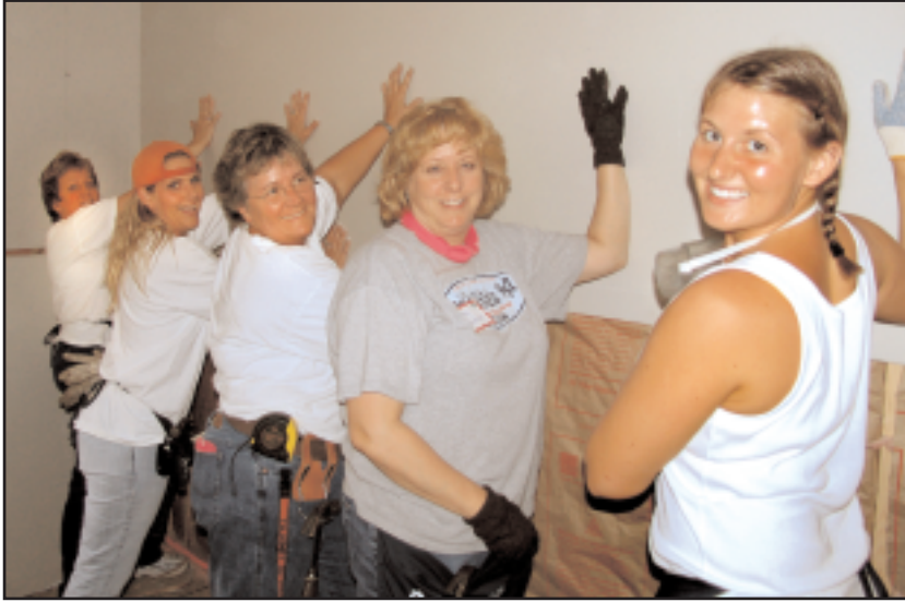
Cindy Bormuth, Deb VanAtta, Linda Fielder, Penny Gerdeman and Heather Martin hang dry wall for Habitat for Humanity.
